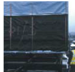
Modules located on steel grillage.
